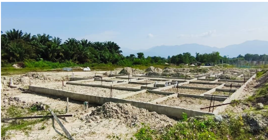
Phase 4B, 1-Storey Terrace Houses, Taman Impiana Bidor, Perak. (Construction works in progress)
