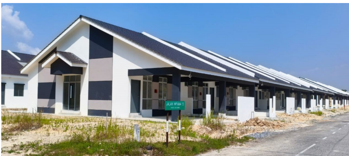
Phase 2B, 1-Storey Terrace Affordable Houses, Taman Impiana Bidor, Perak. (Construction stage at 72.5% and CCC is expected to be obtained in the third quarter of 2026)
