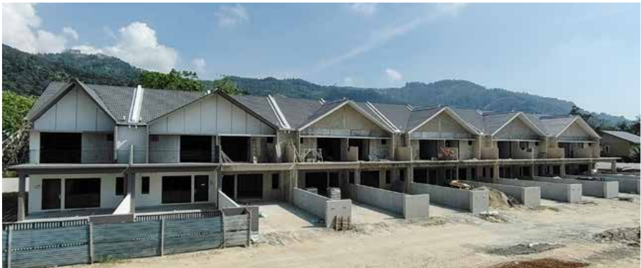
2-Storey Terrace Houses, Taman Impiana Upeh, Balik Pulau, Penang. (Construction works in progress)
